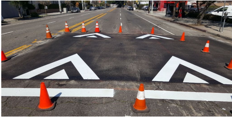
Photo 27 Construction of a “speed table,” an elongated speed hump designed to more reduce traffic speed while maintaining traffic flow
